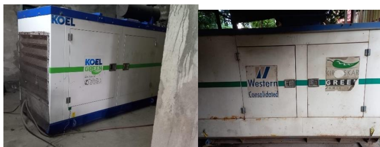
Fig: Green generator sound proof
